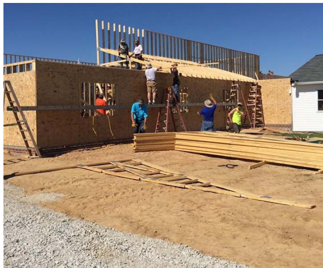
This is the construction scene at New Hope Baptist Church, Dyer. Several Christian based volunteers have come in to help from other states.
